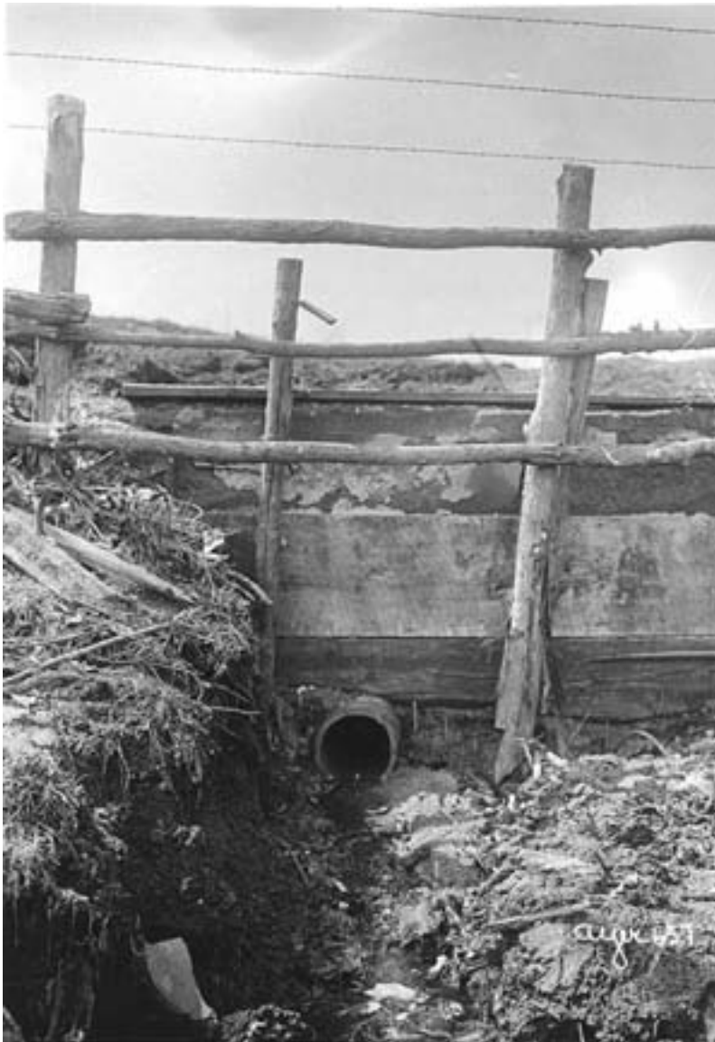
This drain tile required structural support at its outlet to the ditch. Location unknown, circa 1910. (MHS photo by Harry Darius Ayer)
