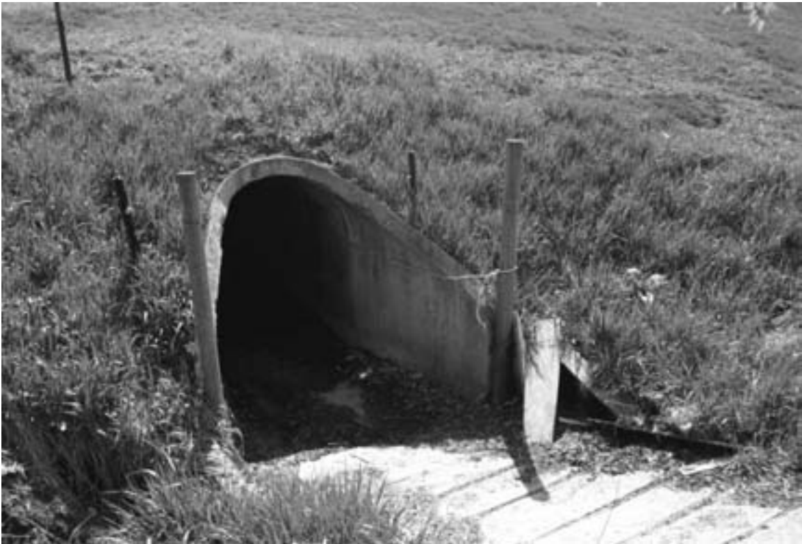
This poured concrete animal underpass in central Minnesota is approached by a scored concrete walkway. The walkway provides traction for animals and reduces erosion on the steep slope. Stearns County, 2004. (Gemini Research photo)
