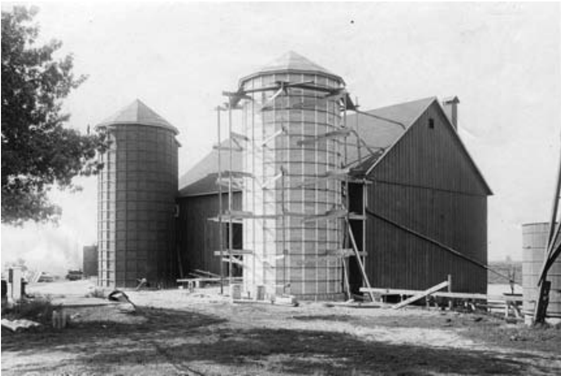
Some horizontal wooden silos were reinforced with vertical boards and then a set of iron bands. This silo, which had both vertical boards and bands, was under construction. Blackinere Farm near Albert Lea, circa 1910. (MHS photo by Harry Darius Ayer)
