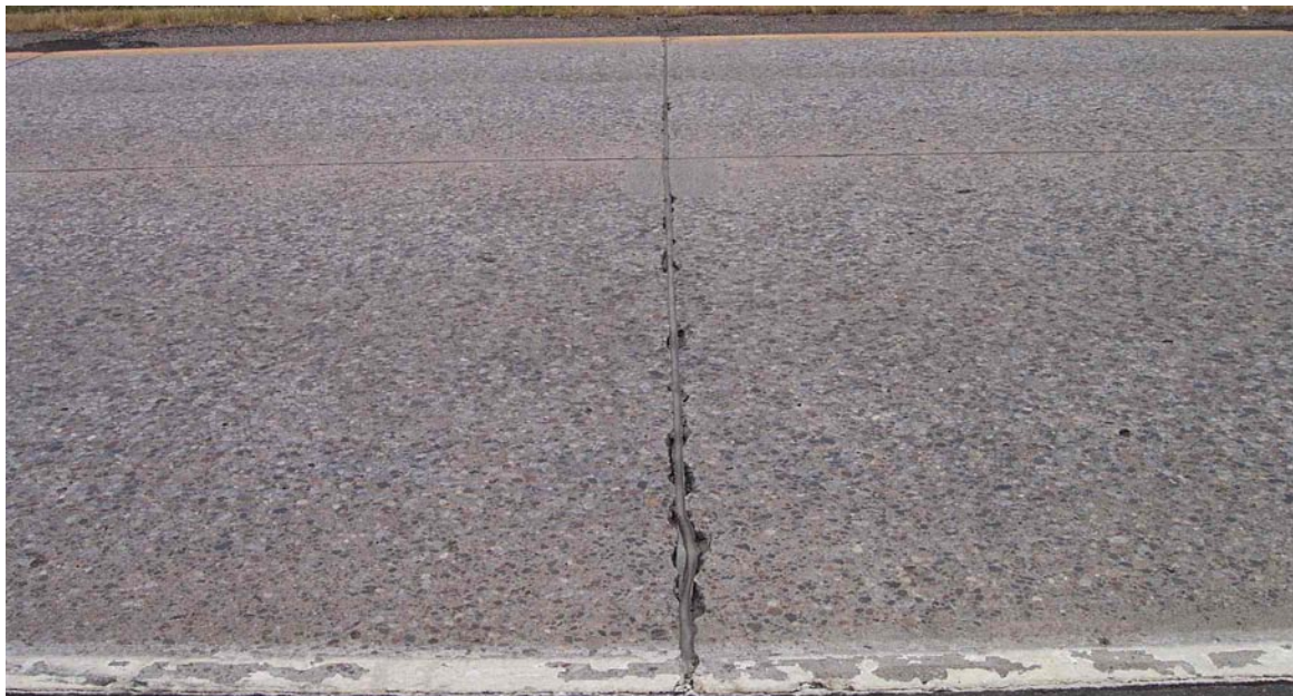
Figure 25. Low Severity Transverse Joint Spalling
