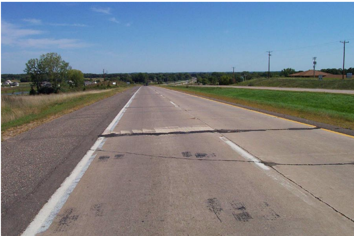
Figure 33. Cracked Panel (slab is divided into two pieces)
