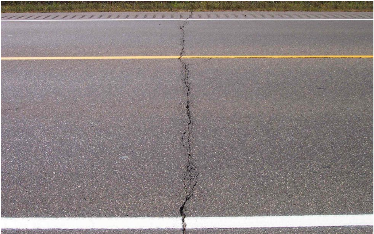
Figure 5. Medium Severity Transverse Crack (some spalling and random cracks)
