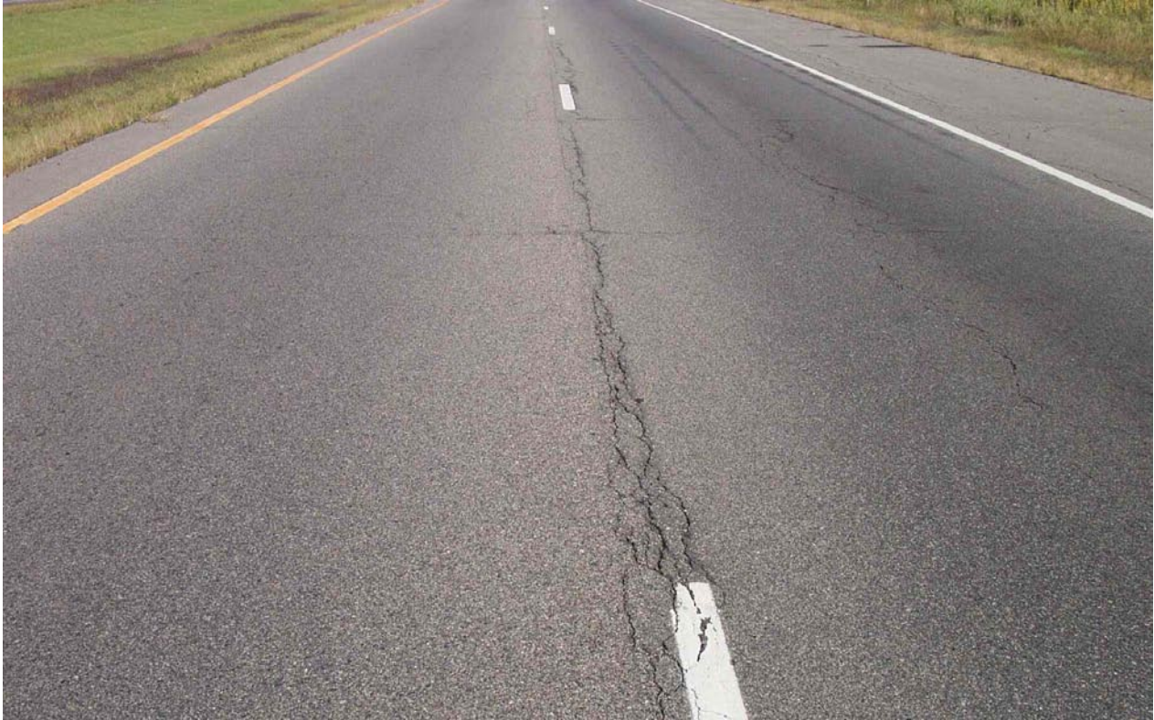
Figure 14. Medium Severity Longitudinal Joint Deterioration (random cracks)
