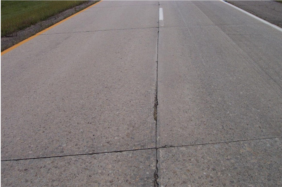
Figure 27. Low Severity Longitudinal Joint Spalling
