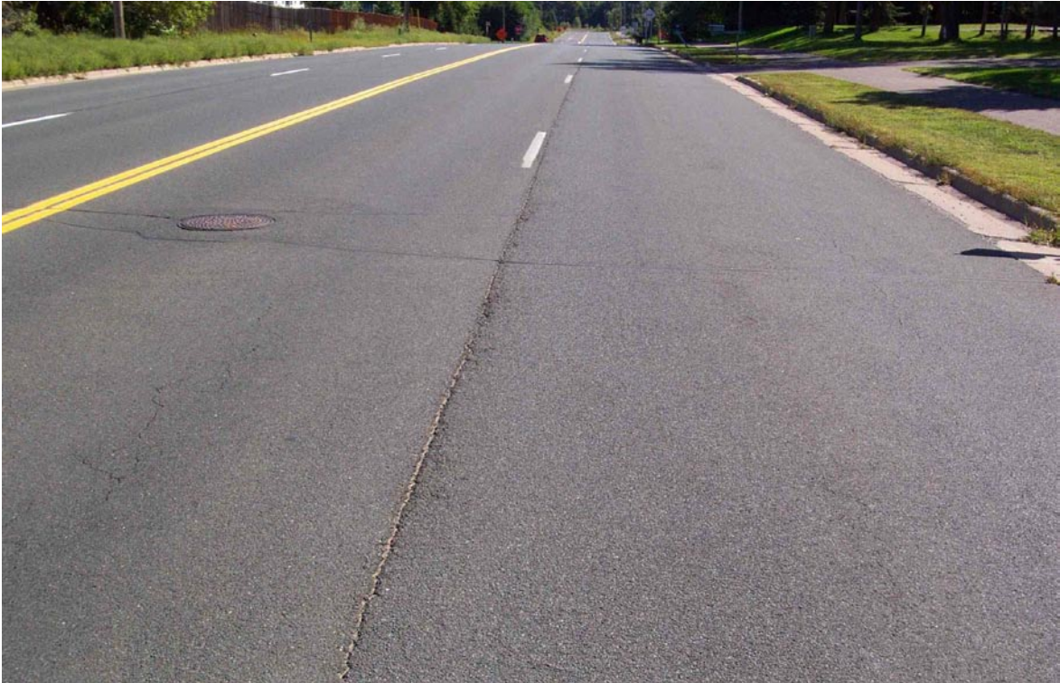
Figure 12. Low Severity Longitudinal Joint Deterioration (no spalling or random cracks)
