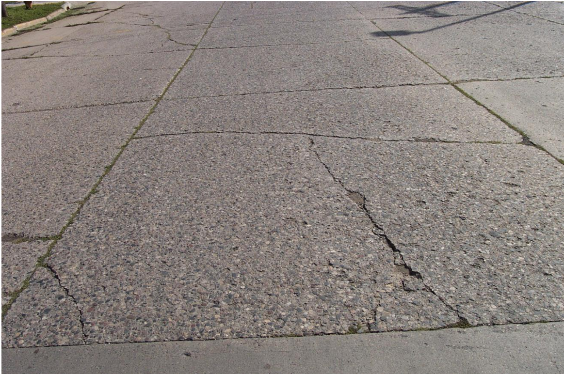
Figure 35. Cracked and Broken Panel
