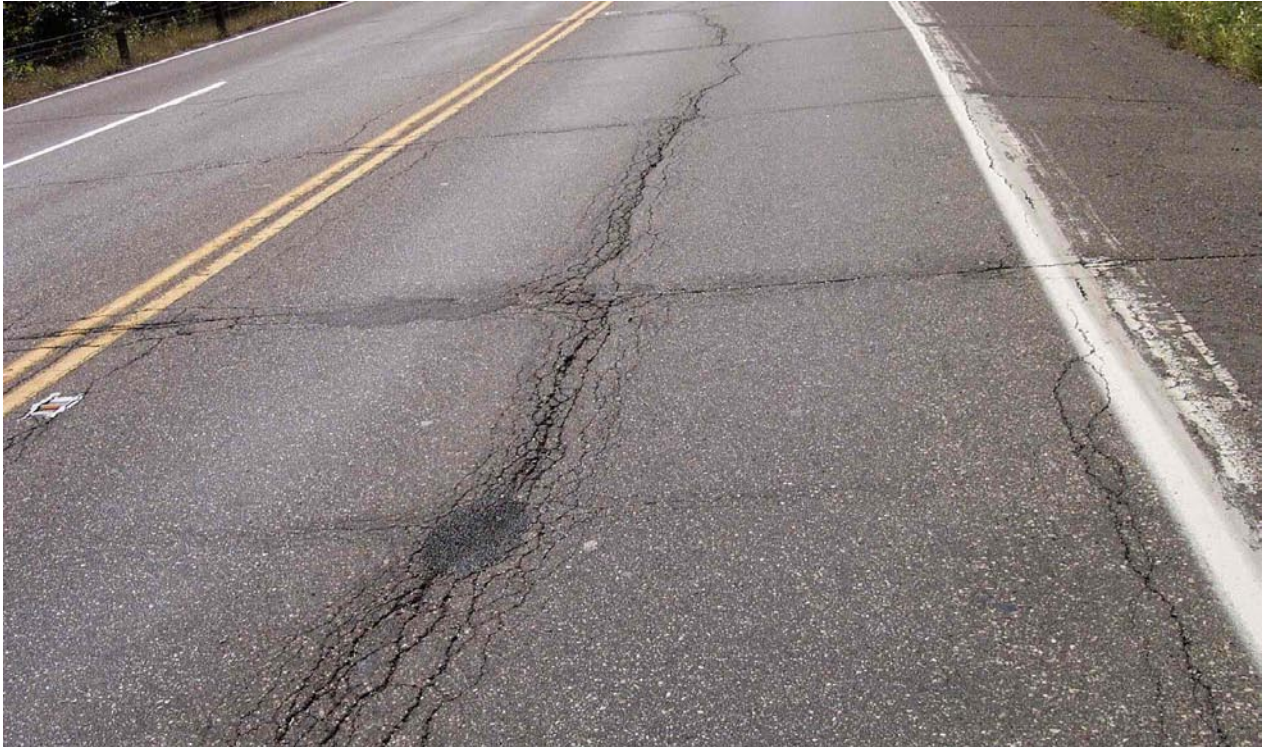
Figure 11. High Severity Longitudinal Crack (random cracks over 12” wide)
