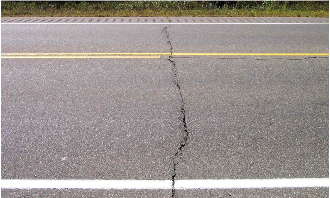
Figure 4. Medium Severity Transverse Crack (some spalling and random cracks)
