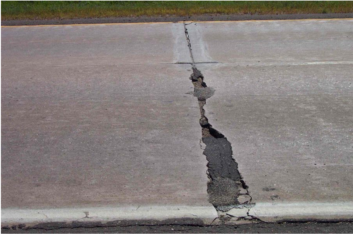
Figure 30. High Severity Transverse Joint Spalling
