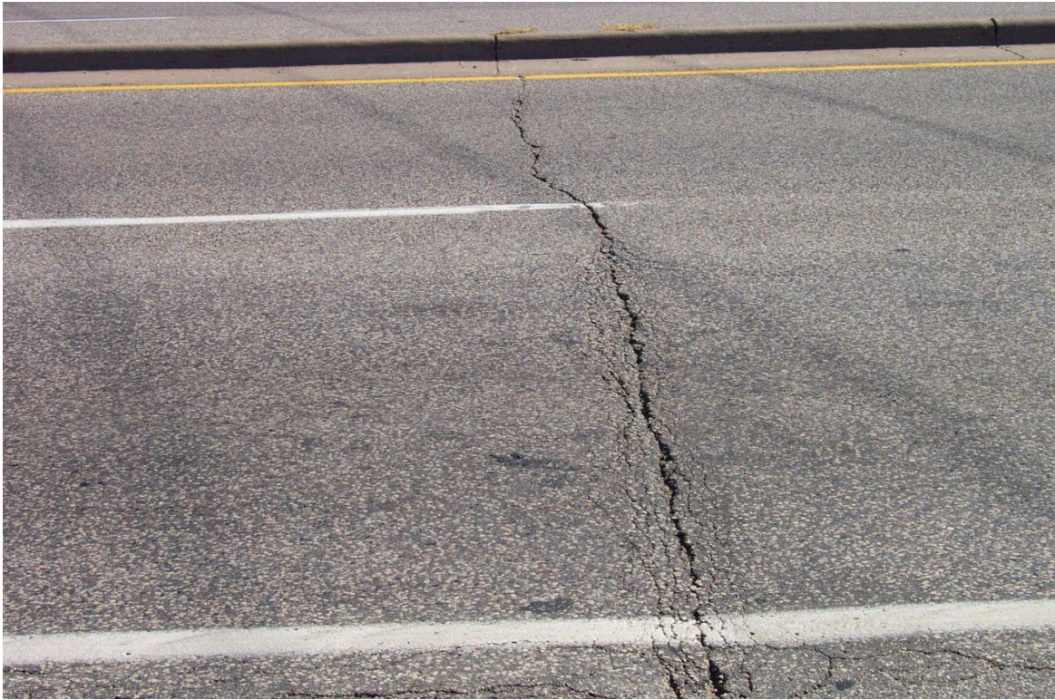
Figure 6. High Severity Transverse Crack (random cracking over 12" wide)
