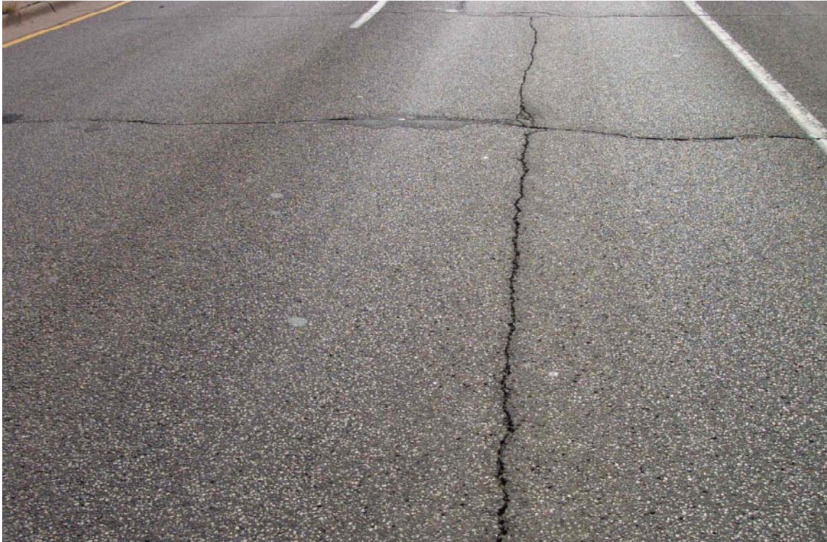
Figure 9. Slight Longitudinal Cracking (no spalling or random cracks)
