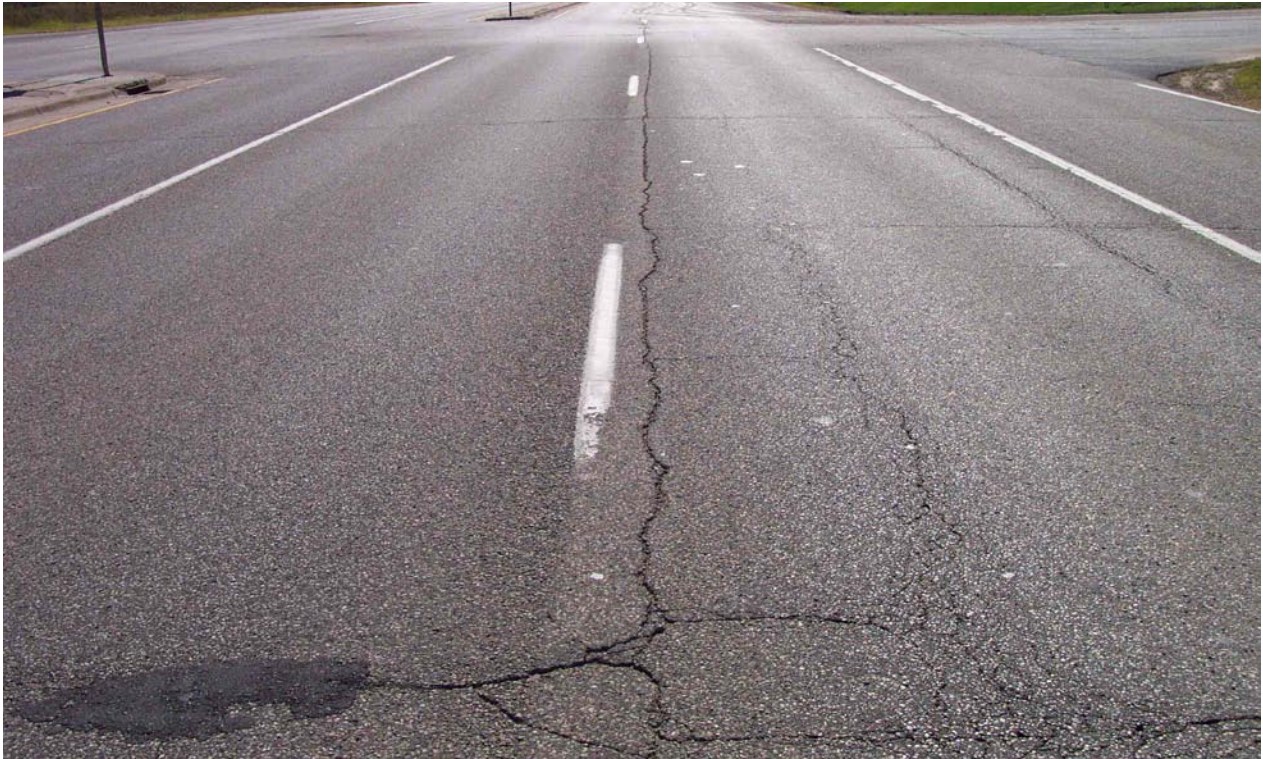
Figure 13. Low Severity Longitudinal Joint Deterioration (no spalling or random cracks)
