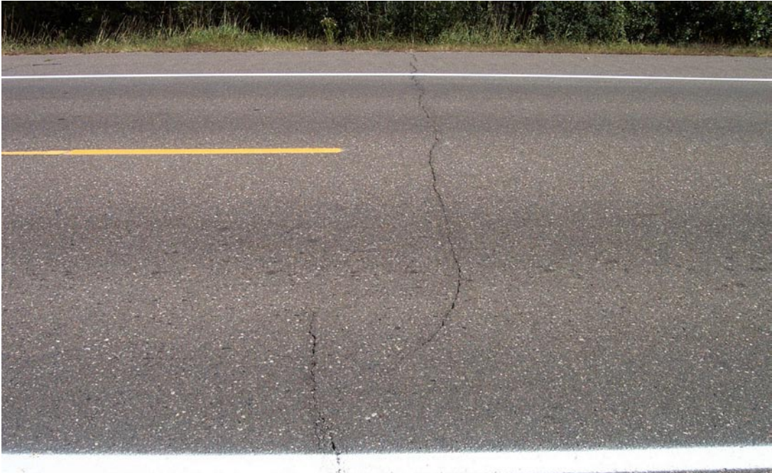
Figure 1. Low Severity Transverse Crack (no random cracks)
