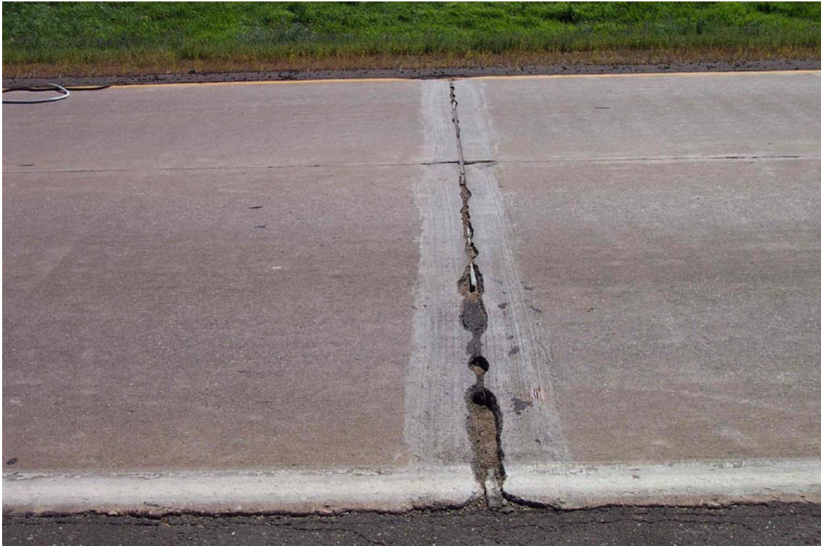
Figure 29. High Severity Transverse Joint Spalling
