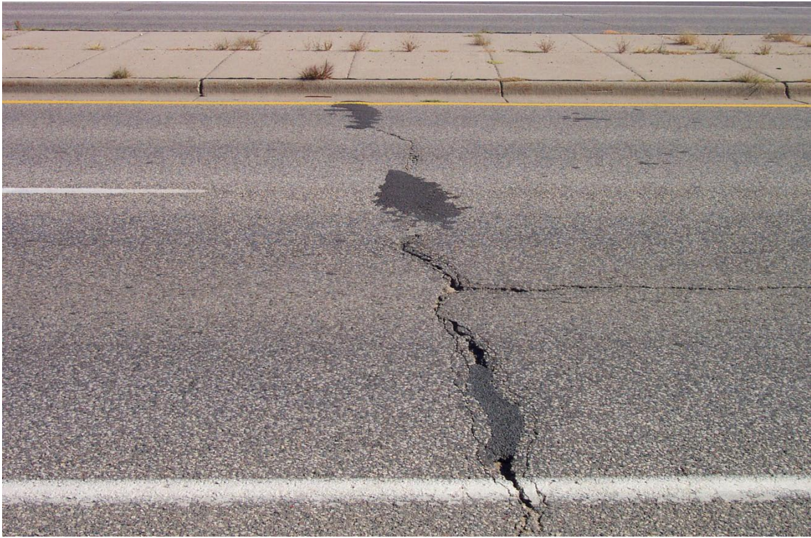
Figure 7. High Severity Transverse Crack (spalling and missing pieces)
