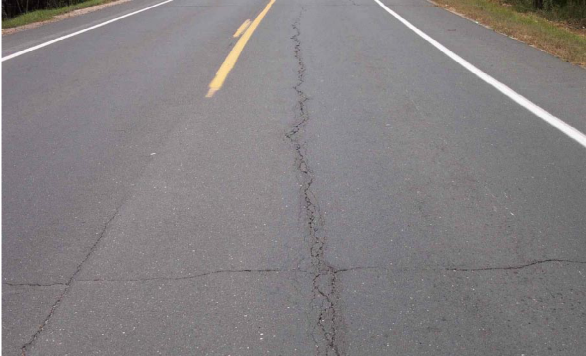
Figure 10. Medium Severity Longitudinal Crack (random cracks are less than 12" wide)
