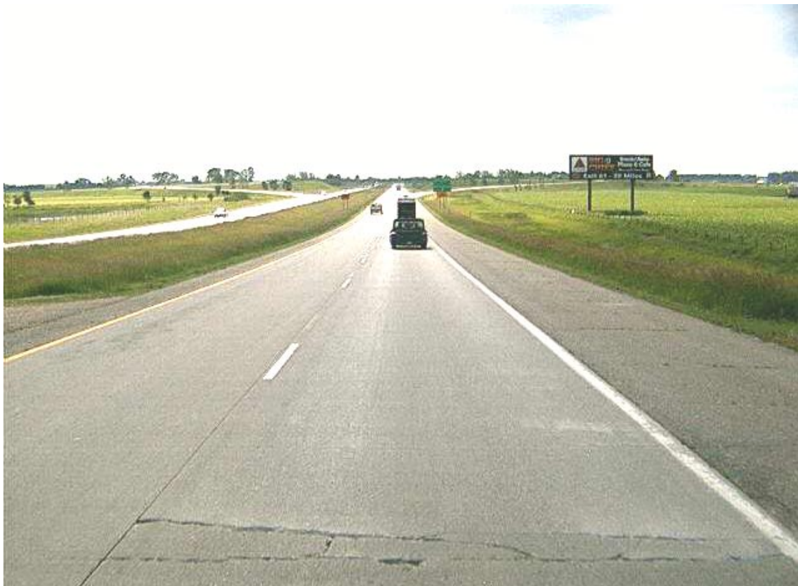
Figure 47. Transverse Crack on CRCP
