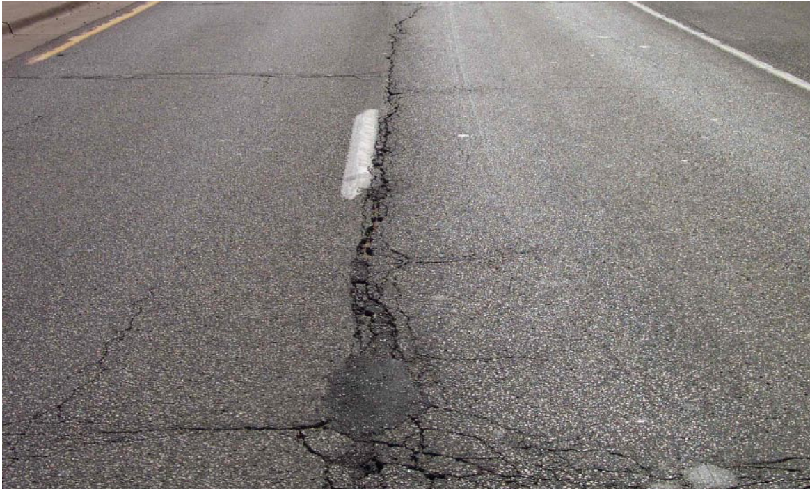
Figure 16. High Severity Longitudinal Joint Deterioration (spalling)
