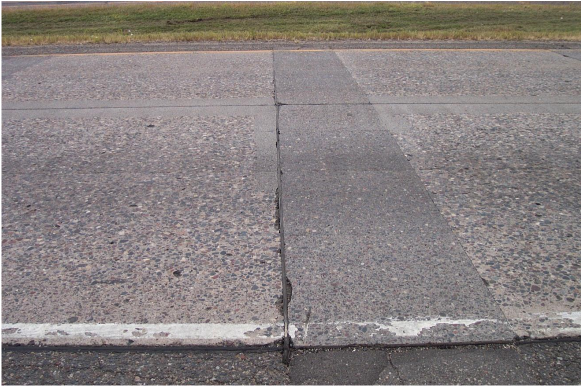
Figure 26. Low Severity Transverse Joint Spalling
