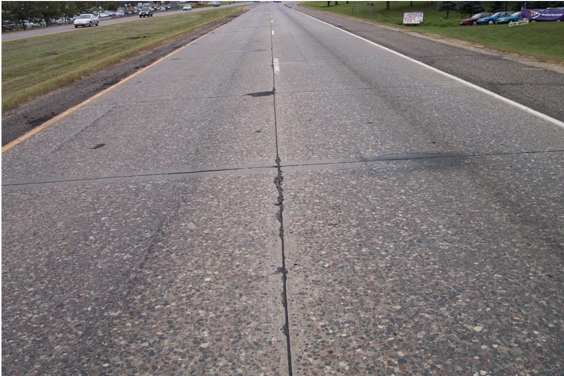
Figure 28. Low Severity Longitudinal Joint Spalling
