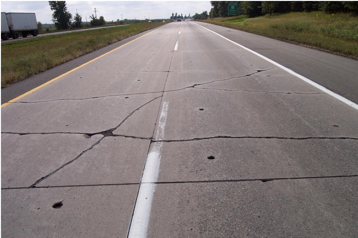
Figure 36. Cracked and Broken Panel
