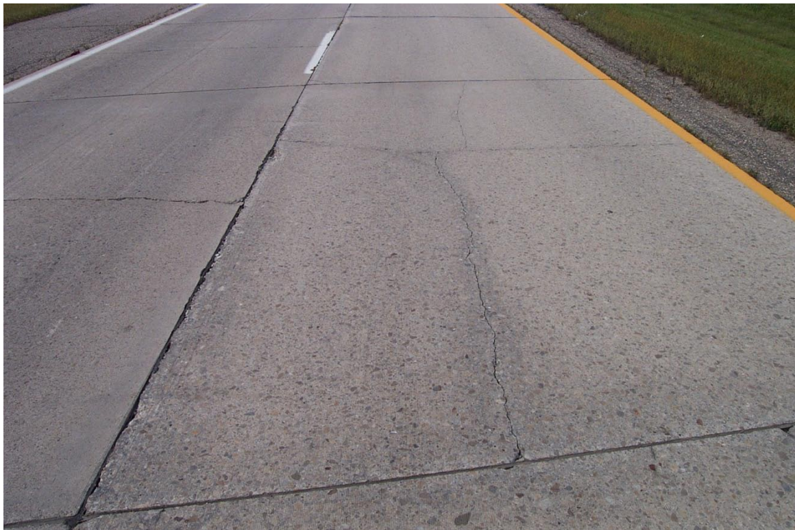
Figure 34. Cracked and Broken Panel
