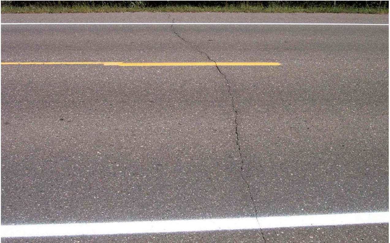
Figure 2. Low Severity Transverse Crack (no random cracks)
