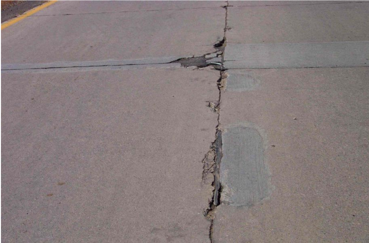
Figure 31. High Severity Longitudinal Joint Spalling
