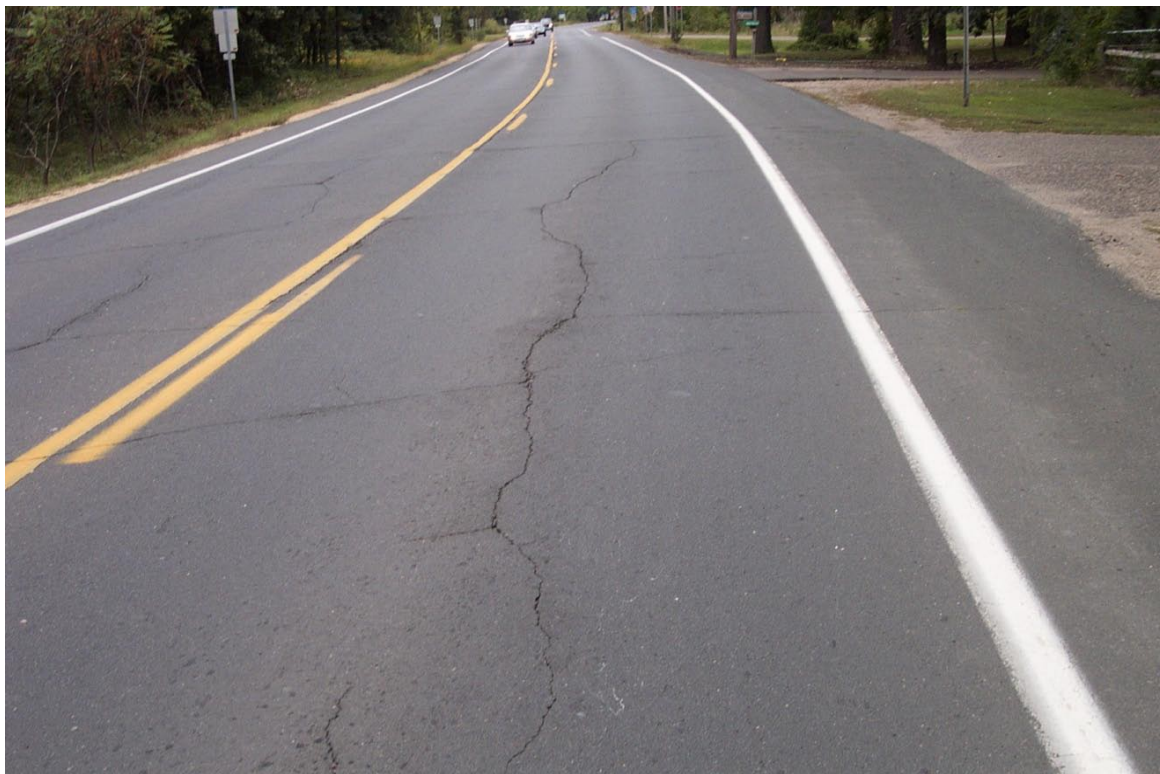
Figure 8. Low Severity Longitudinal Crack
