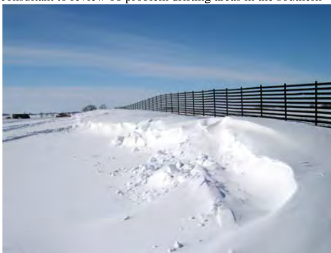
Figure 6-4. Structural Snow Fence
