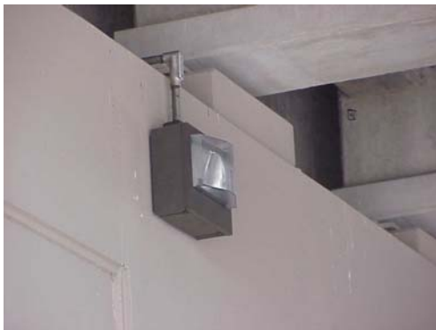
Bridge Underpass Luminaire
