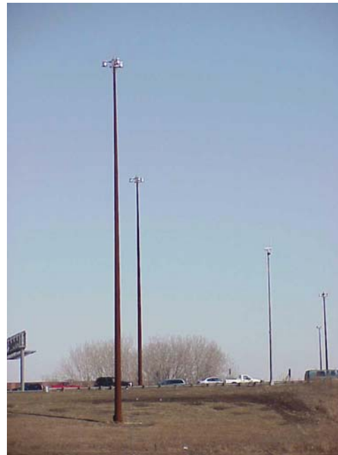
High Mast Tower Poles (3-100, 4-100, etc.)
