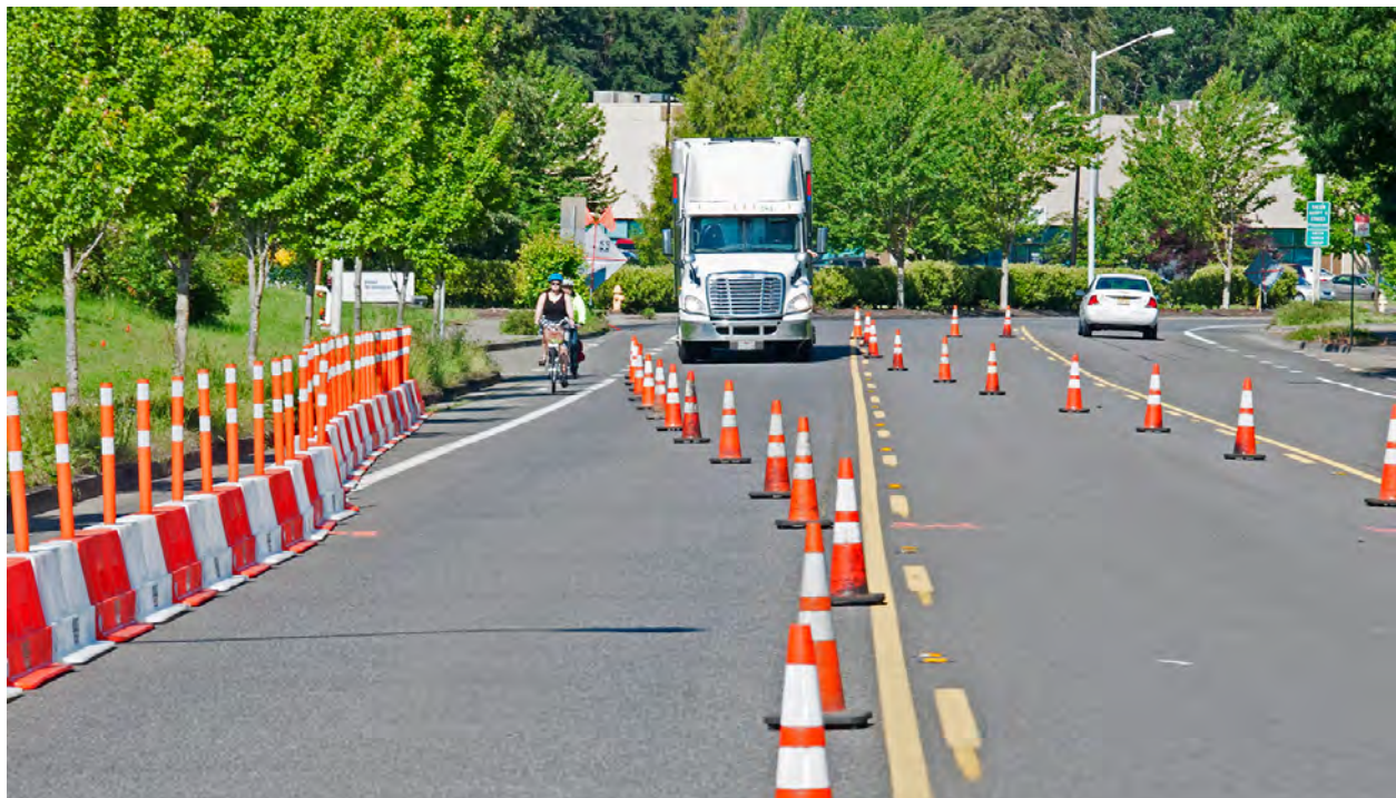
Figure 1: Example of bicycle facility maintained through work zone (source: Oregon Department of Transportation)
