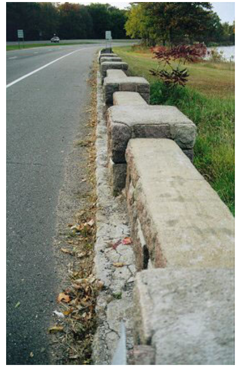
7. North end of West side Wall (Note: condition of curb and mortar)
