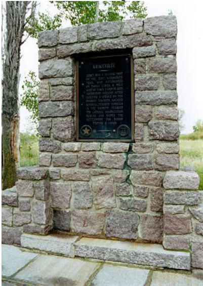
3. South View of Marker (note: stone joint deterioration)
