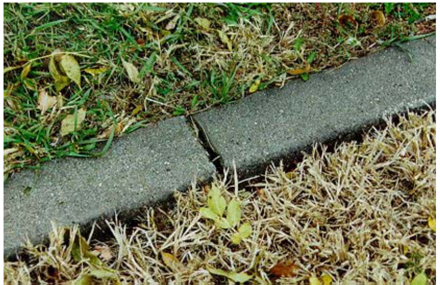
15. Close-up of Concrete Curb showing overgrown turf
