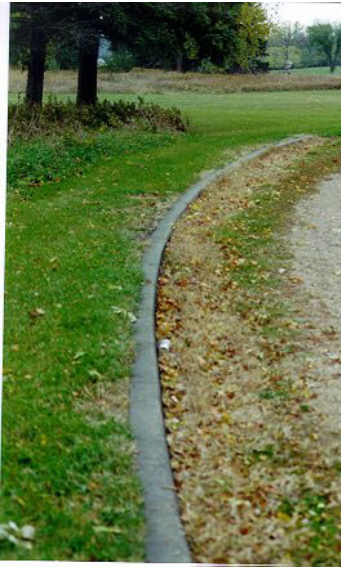
14. Curb & Drive looking East (Note: overgrown turf)
