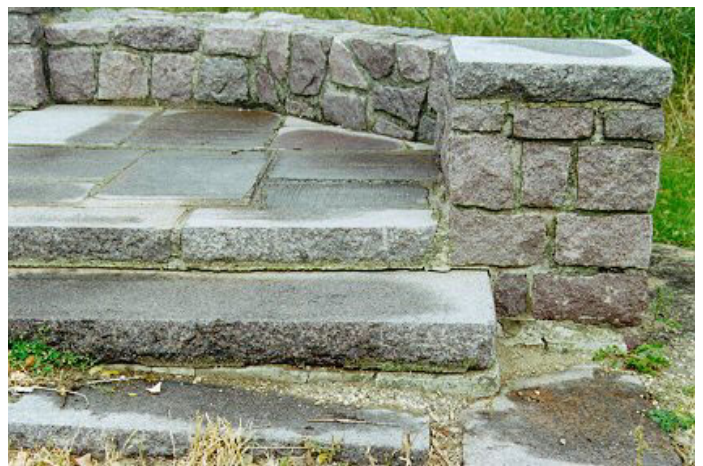
13. East End of Marker Steps (Note: joint conditions, mortar cracks and invasive turf)
