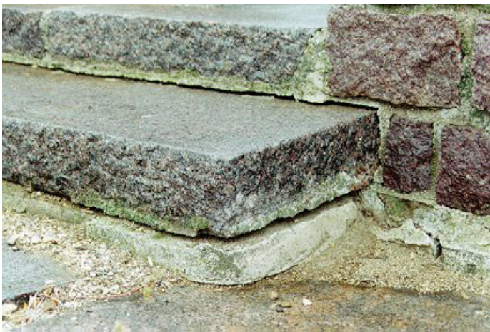
10. Granite step at East End (Note: grade settlement from excess mortar fill)
