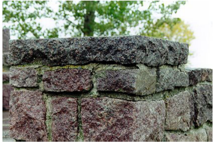
9. Close-up of Pier (Note: spalled cap stone and decaying mortar)
