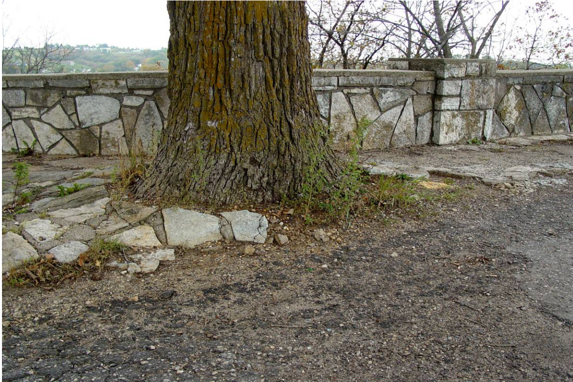
Plate 14. Disruption of flagstone terrace by tree growth, facing south
