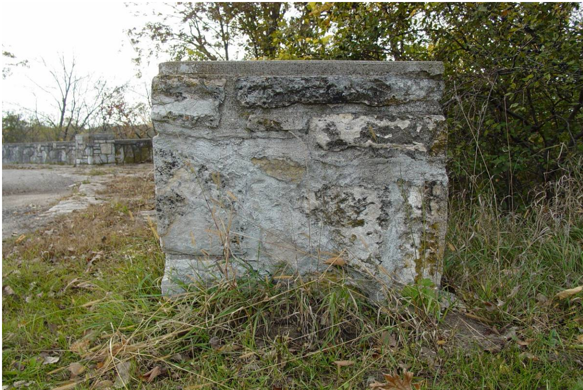
Plate 5. Improper repointing on western pier of overlook wall, facing east
