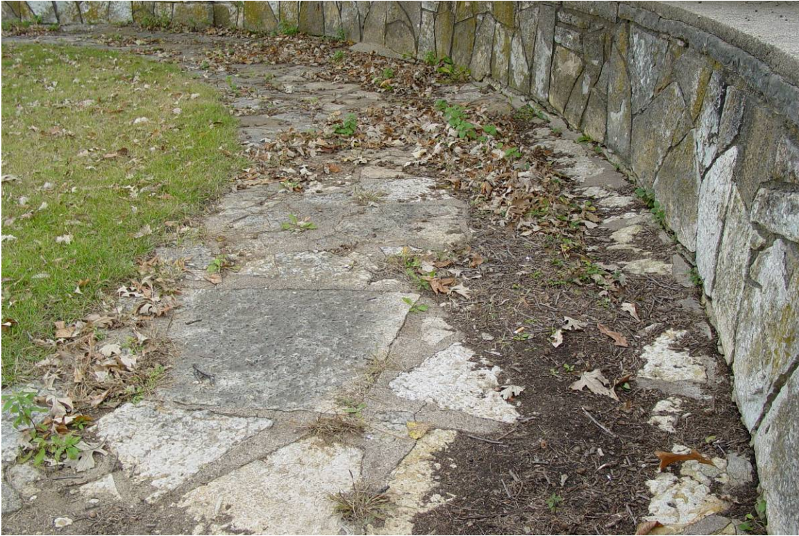
Plate 12. Subsidence of flagstone terrace adjacent to overlook wall and gravel island, facing east
