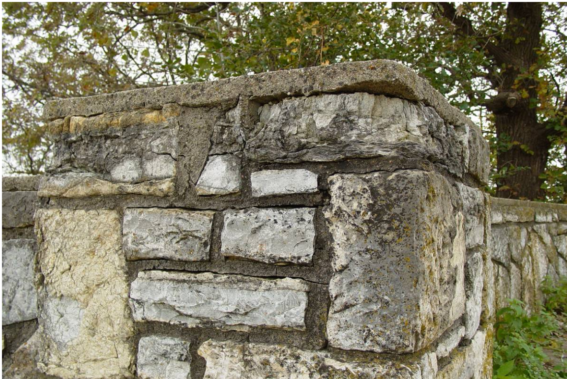
Plate 7. Deteriorated stone in pier near central portion of overlook wall, facing southwest
