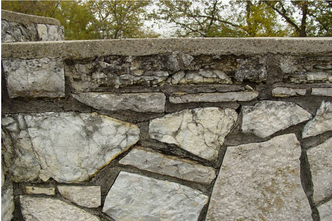
Plate 8. Deteriorated stone in overlook wall, facing east
