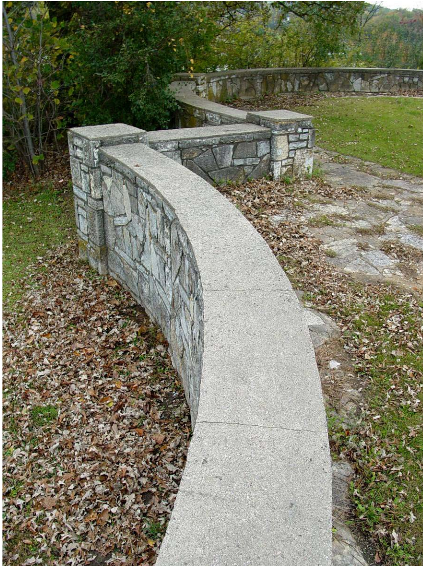
Plate 16. Cracks in concrete cap at east end of overlook wall, facing south
