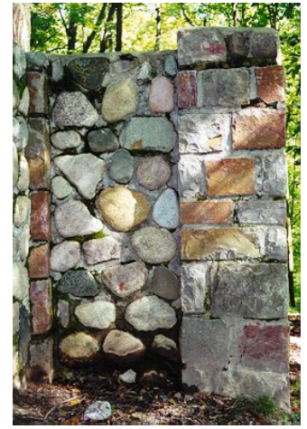
15. View of lower wall condition.
