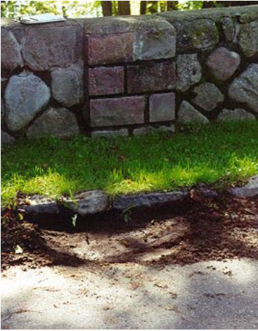
22. Original catch basin covered with asphalt overlay.
