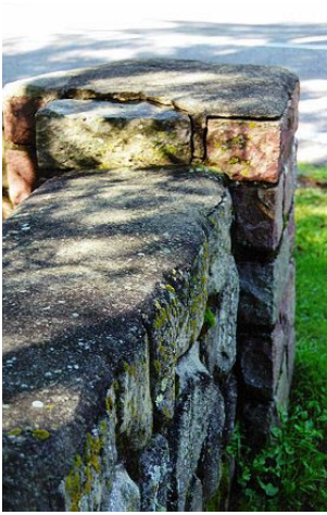
13. Existing mortar cap condition
