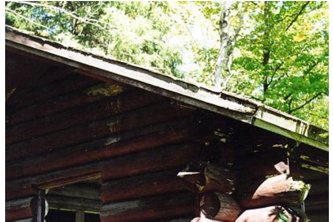
6. Fascia/shingle and log end deterioration.
